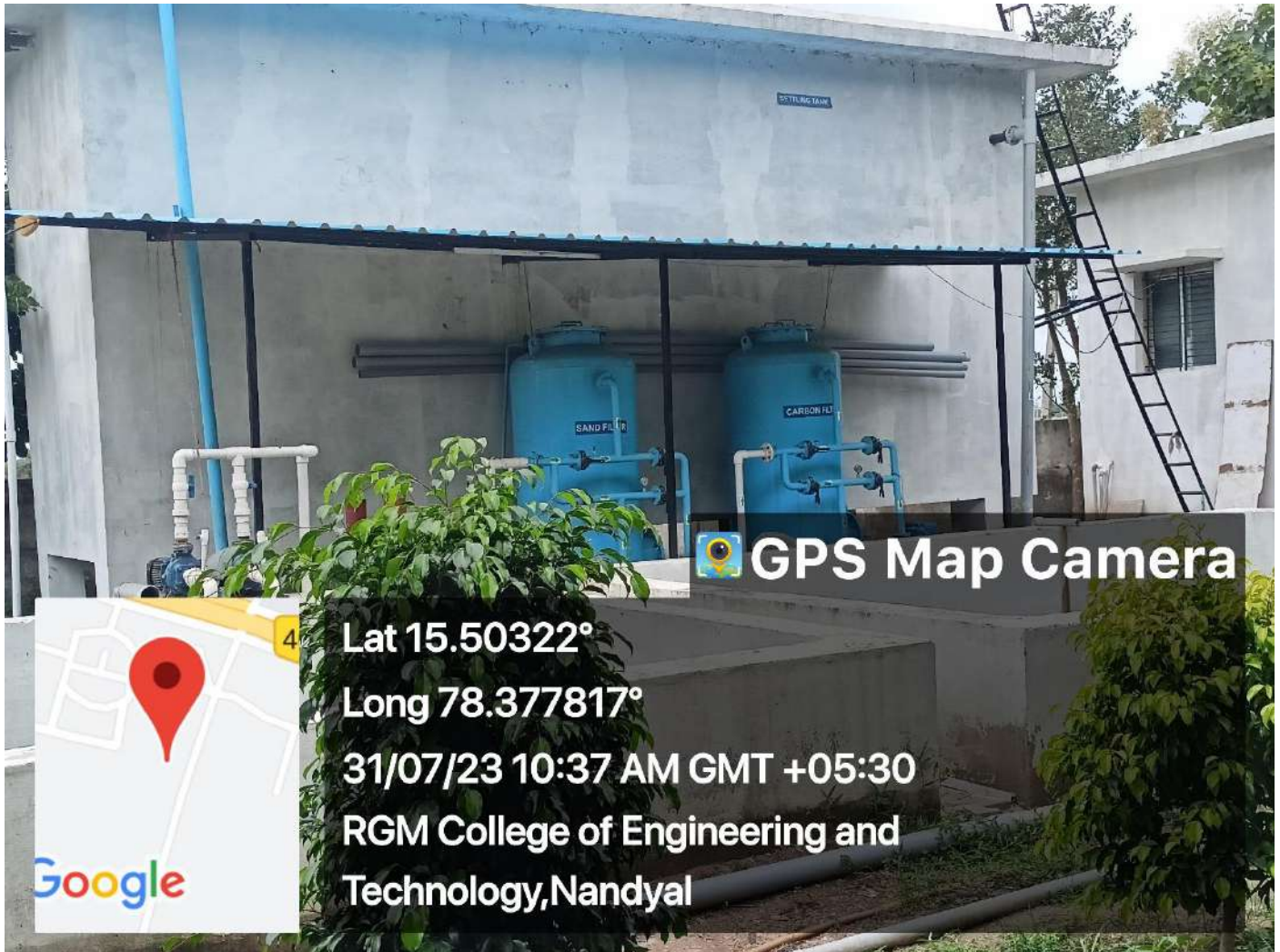
Waste Water Recycling Plant in front of ME Block
