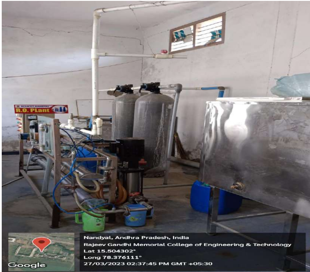
R O Water Plant in the Campus
