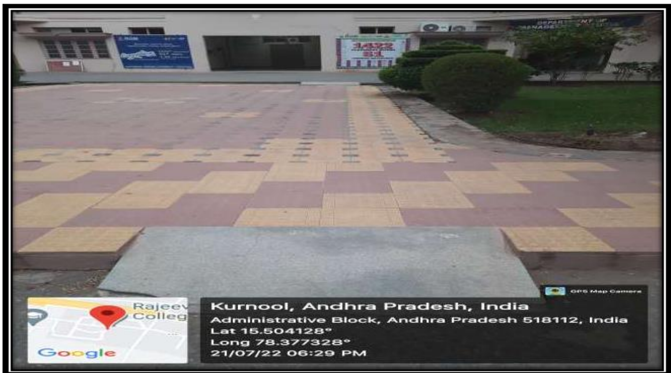
Pedestrian friendly Pathways having Ramp facility
